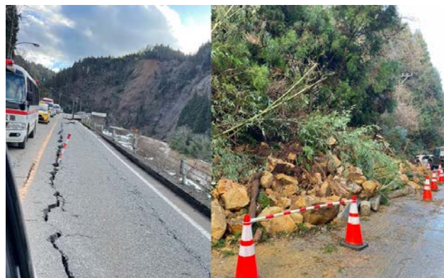
The roads on the way to the Noto Peninsula have suffered severe damages due to extreme changes in terrain.
